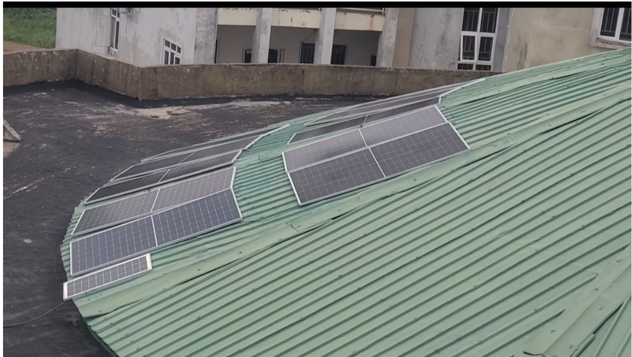
Figure 3.3: Solar Panel Array on Rooftop
