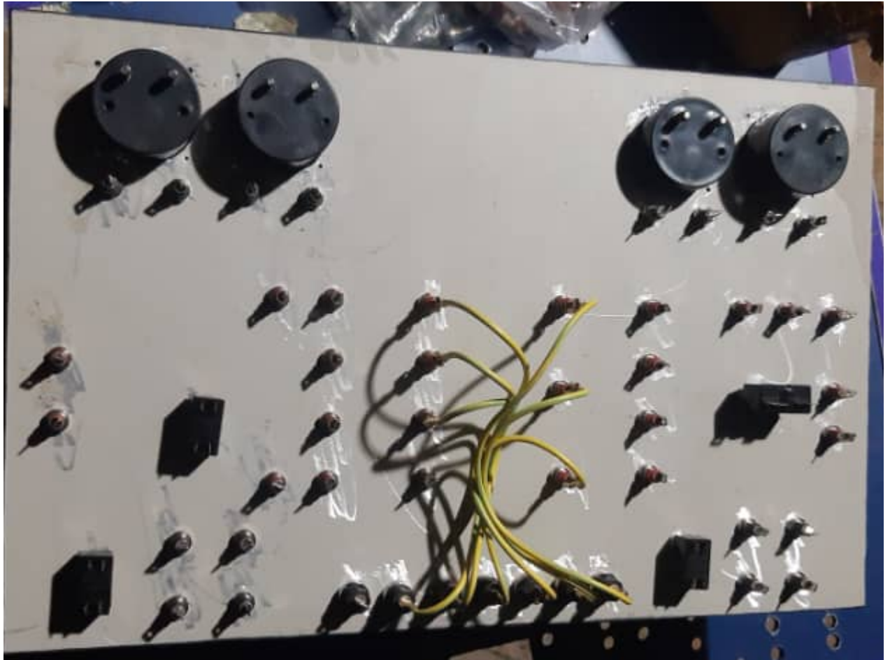
Figure 3.5: Transformer circuit board internal connection
