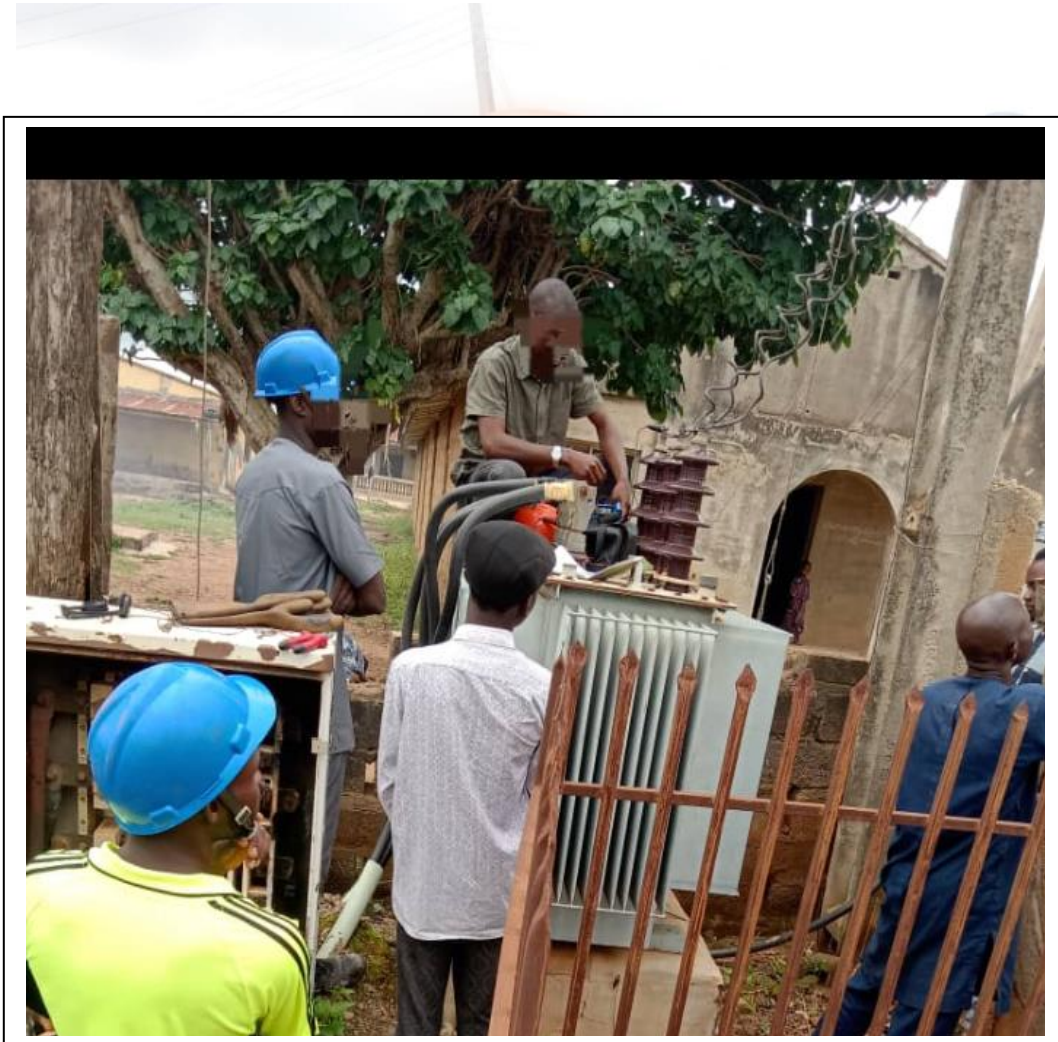
Bi-annual Maintenance at injection substation
