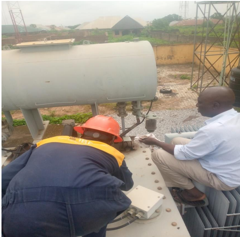
Checking the oil level at injection substation
